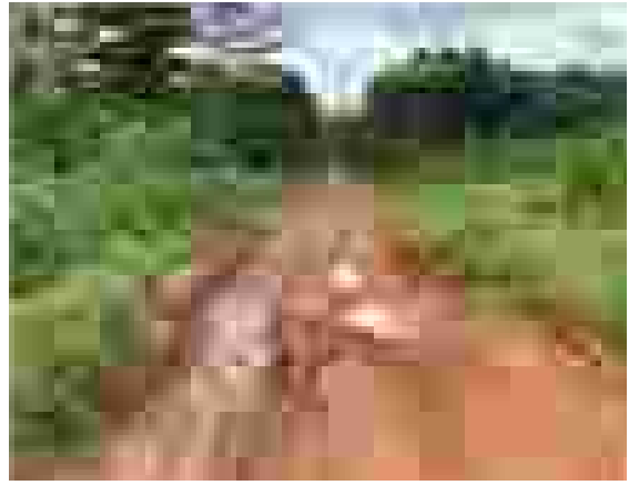
Figure 1-3: Potholes, Puddles and gullies which make the road impassable during the rainy season.
