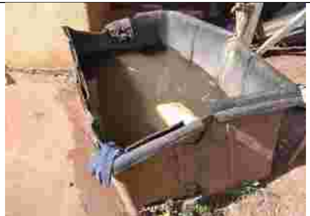
Figure 17: Sanitary Facility water storage tank
